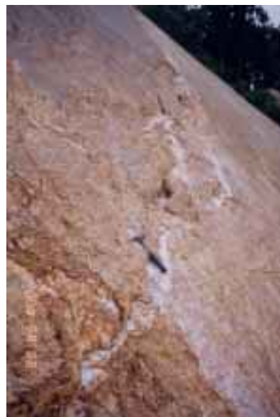
Photo.10 White clay adhered to joint of granite Yamaguchi-shi in Yamaguchi Prefecture
