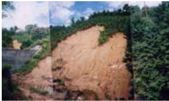
Photo.7 Slope failure consisting of granite at Hiroshima-shi in Hiroshima Prefecture
