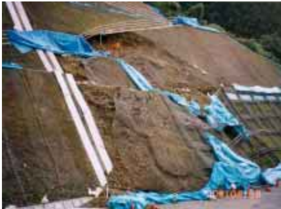
Photo.11 Slope failure of Sangun metamorphic rock at Tokuyama-shi in Yamaguchi Prefecture
