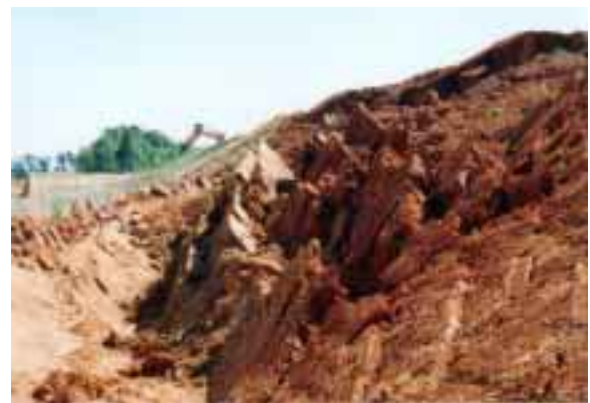
Photo.5 Toppling failure of slope consisting of Sangun metamorphic rock at Ube-shi in Yamaguchi Prefecture
