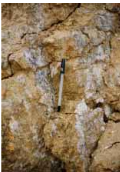
Photo.9 White clay adhered to joint of granite at Higashiroshima-shi in Hiroshima Prefecture
